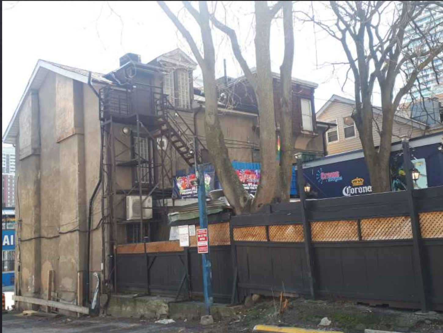
Looking Southeast at North (Side) and West (Rear) elevation of 508-510 Church Street, Toronto: May 2020 39
