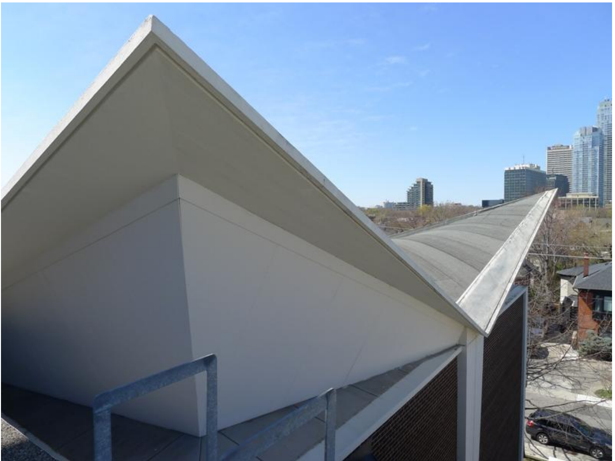
18. Central Entry Pavilion Roof – side view : showing the side elevation and a portion of the edge of the central roof. (HPS, 2016)
