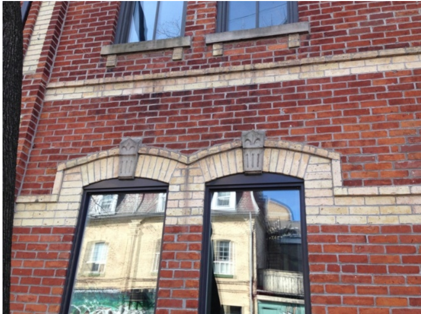
11. Vogon Block, East Elevation, showing the details of the windows including the cast-stone keystone and the details of the upper window sills (HPS, 2017)
