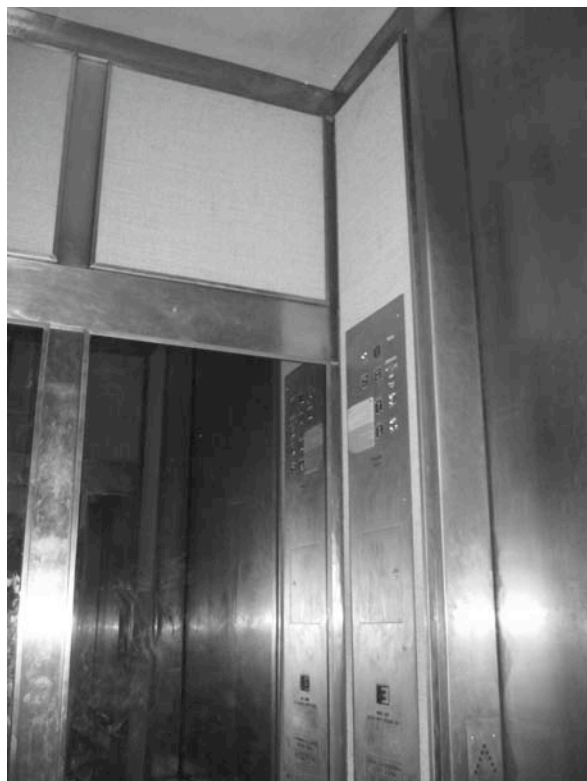
Interior of typical elevator
