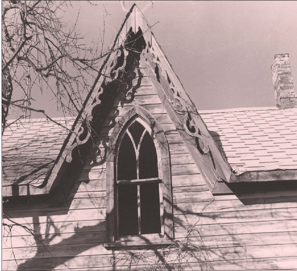
Figure 14 Gothic-style pointed windows and central gables with bargeboards were usual motifs of the symmetrically-planned small-scale house.
