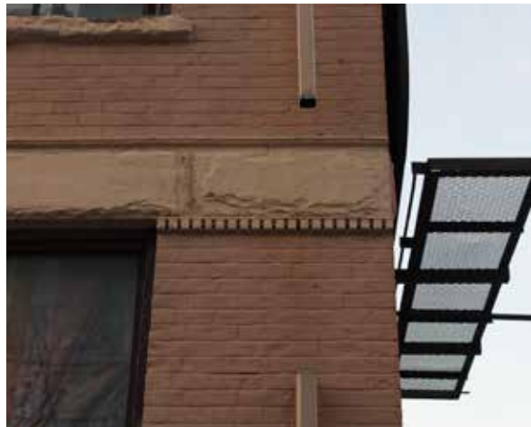
Rainwater systems in poor condition - missing downpipe (ERA, 2017)
