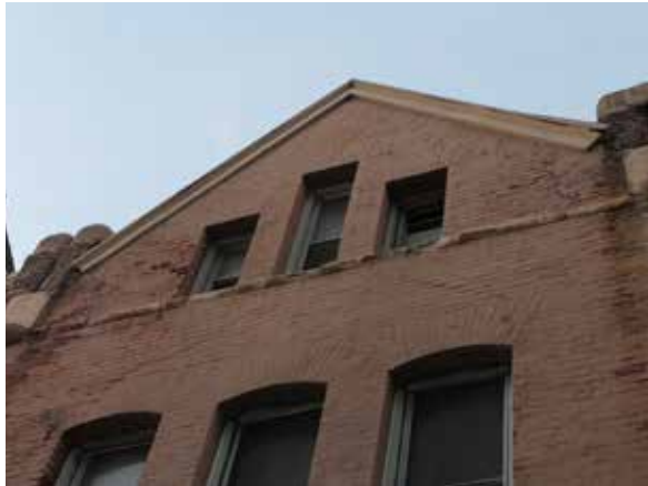
Significant masonry deterioration near the roofline, including spalled bricks and stone sills (ERA, 2017)
