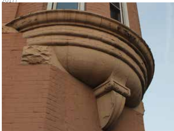
Cut sandstone detailing at corbel in good condition, though heavily overpainted (ERA, 2017)
