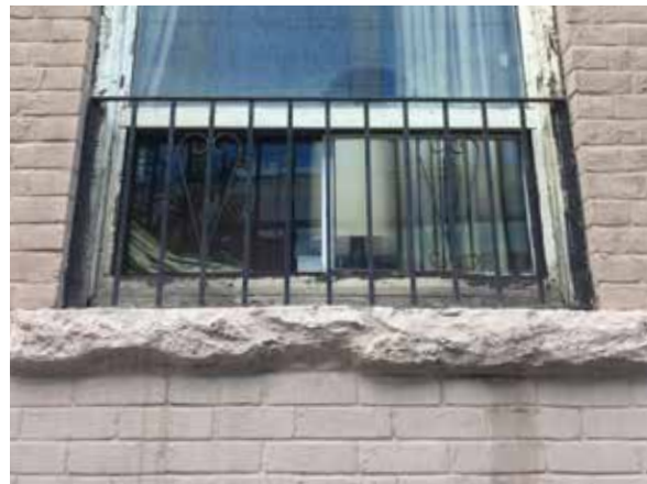
Deterioration of sandstone sill (ERA, 2017)
