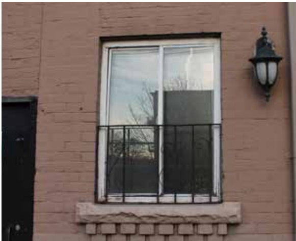
Modern aluminum window units in poor condition - typical (ERA, 2017)
