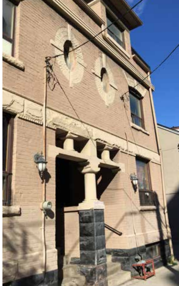
938-944 King Street West, showing masonry in overall good condition, with wear near grade and roofline (ERA, 2017)
