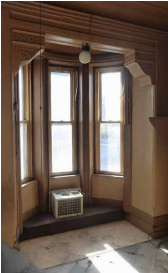
Some interiors retain decorative plaster and millwork in fair condition, 950 King St. W. (ERA, 2017)
