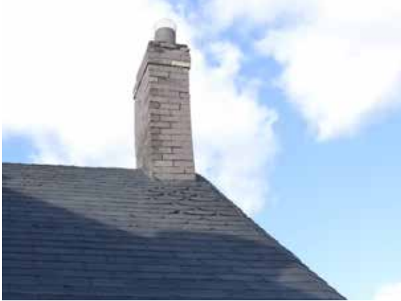
Chimney masonry in poor condition, also showing significant deterioration of asphalt shingles (ERA, 2017)
