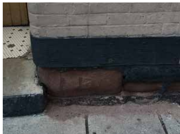
Detail of delamination of sandstone plinth from road salt (ERA, 2017)
