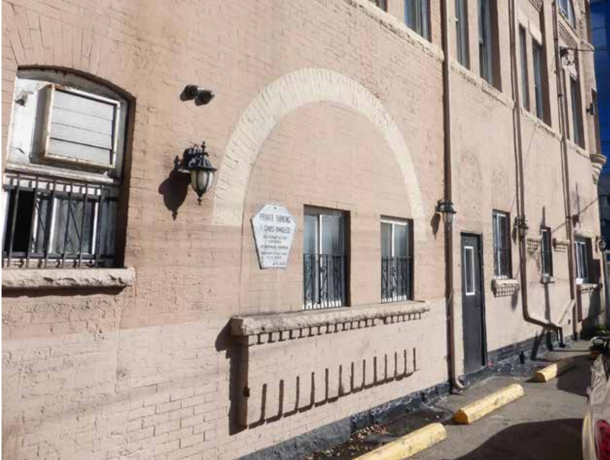
Showing significant modification to openings, bricking-in of arch and modern sealed aluminum window units (ERA, 2017)
