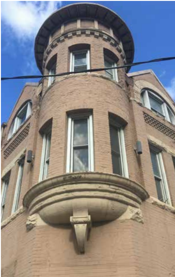
Water damage to masonry visible near the roofline flanking the turret (ERA, 2017)
