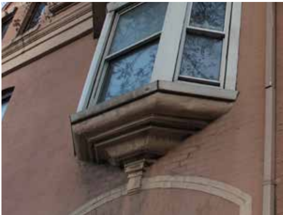
Showing heavy masonry staining under oriel window (ERA, 2017)
