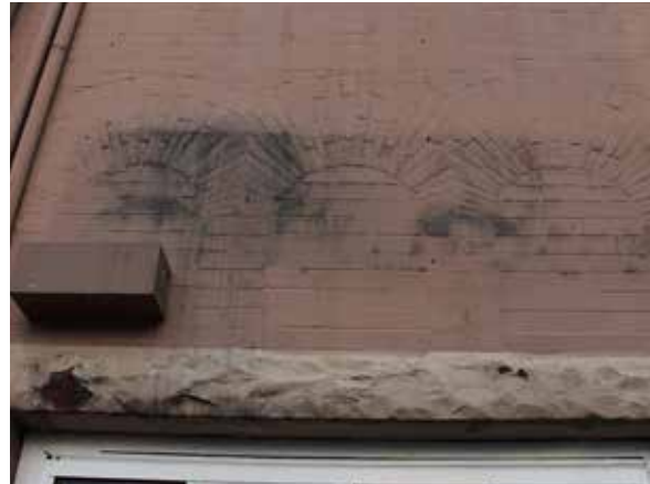
Former openings filled in with brick and signs of environmental staining (ERA, 2017)
