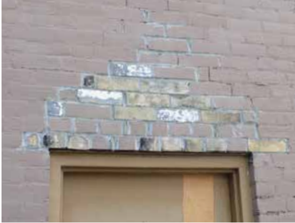
Poorly executed brick repairs (ERA, 2017)
