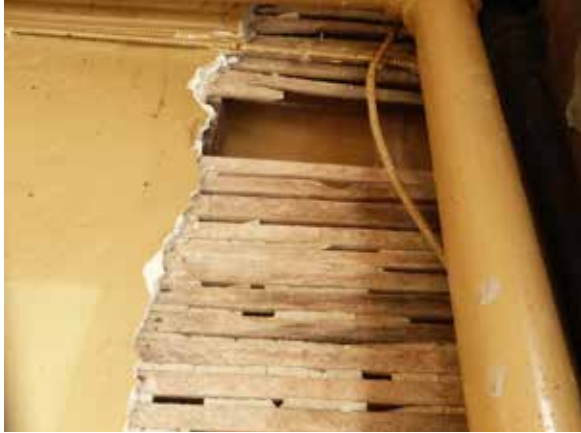
Some interiors in poor condition -- exposed lath & plaster on a partition wall, 950 King St. W. (ERA, 2017)
