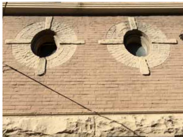
Water staining of brickwork under sills and projections -- typical (ERA, 2017)
