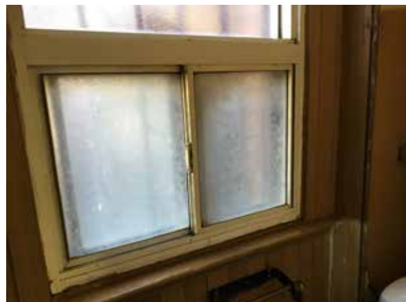
Modern aluminum sealed window units in fair to poor condition -- typical (ERA, 2017)
