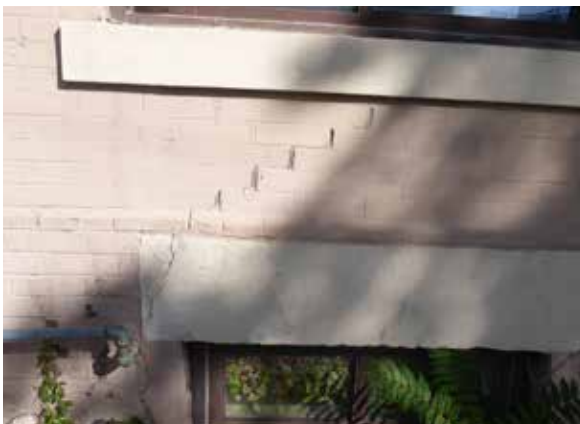
Step-cracking and failed joints revealing settlement of the building (ERA, 2017)
