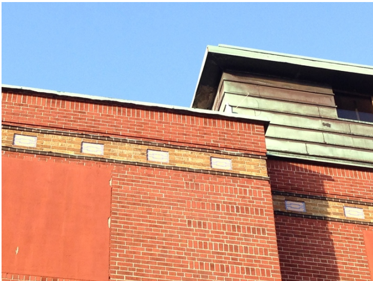
17. Upper level of the south elevation showing the brick detailing and the brick and tile frieze with the copper cladding of the service tower of the former school (HPS, 2018)
